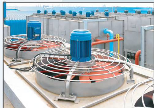
Fan and water pump
